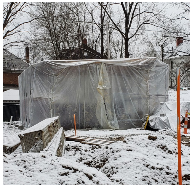
Masonry block and brick are stored within a heated tent to keep the materials above 40°F.
