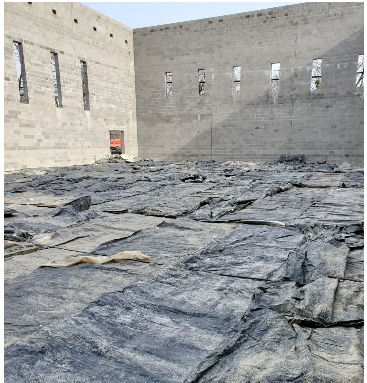
Concrete blankets protect the newly placed concrete slab-on-grade of the gymnasium floor in this new structure.
