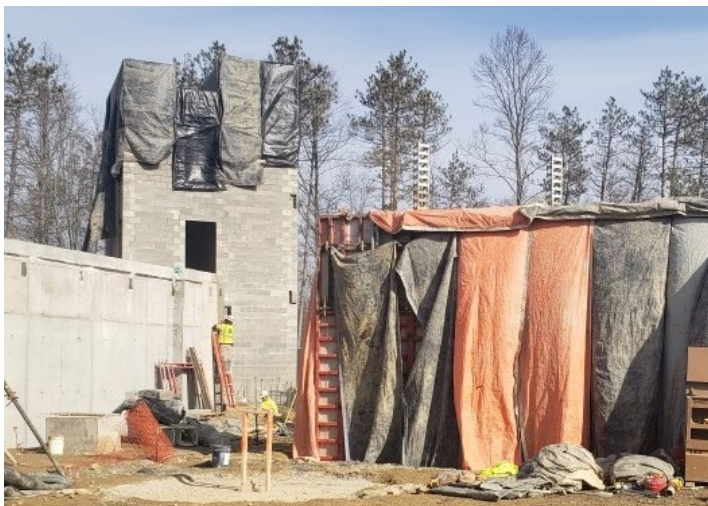
Concrete blankets protect the fresh poured concrete walls and the newly constructed masonry block tower.
