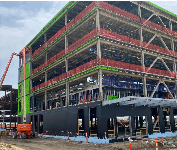
Imaging by drone to support construction observation minimizes technicians' time in precarious situations.
